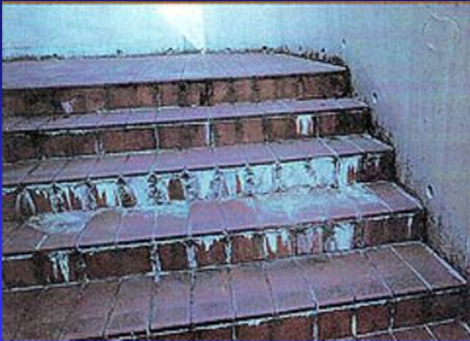
Efflorescence and water damage on brick steps
