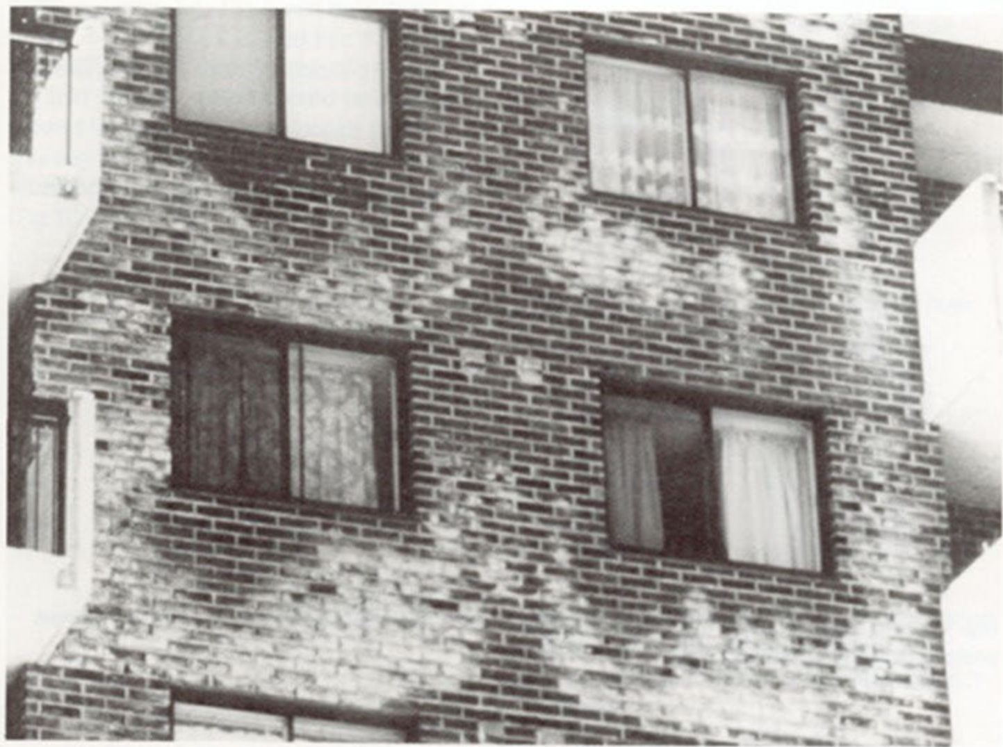
Fig. 16 An example of extensive wetness and efflorescence
