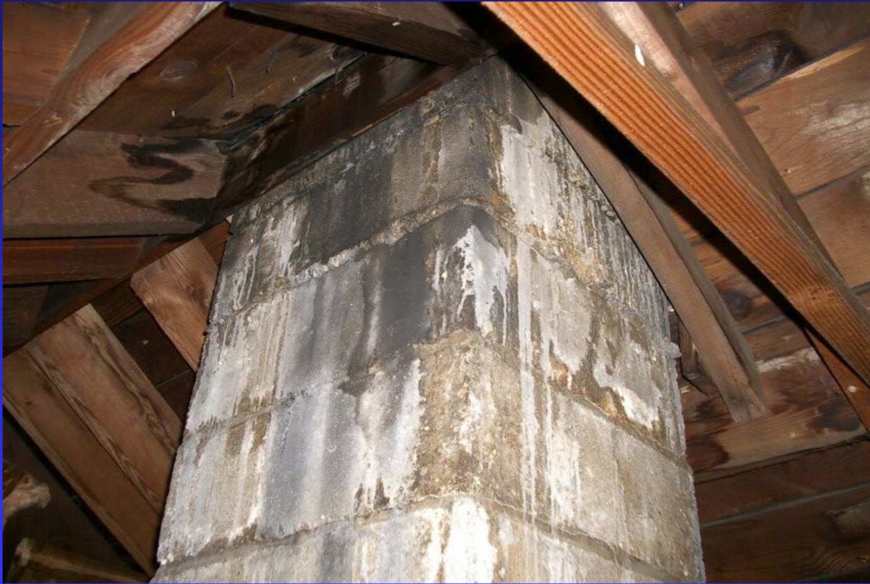
Internal efflorescence and damage due to moisture migration
