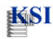
Inlet baffle of same tank as above... photo taken from the outlet side of the tank. That is the inlet pipe extending down into the tank.
